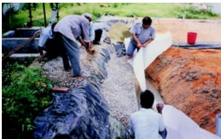
Fig 65. Construction of laying of geotextile and filter media for root zone treatment
